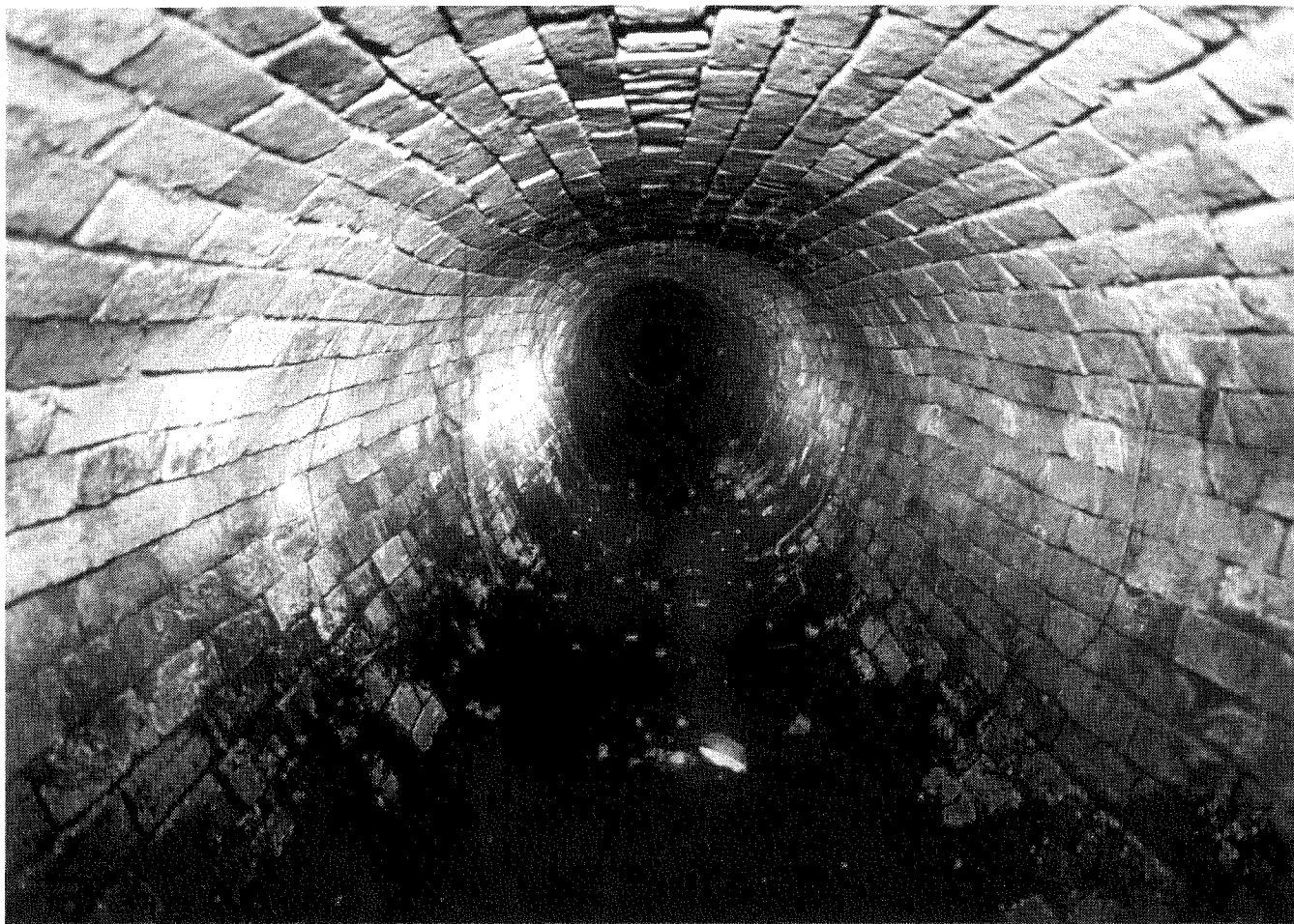
Fig. 3: A section of the complete brick barrel-drain, about 1200mm in diameter, in the vicinity of Phillip Street, Parramatta.
