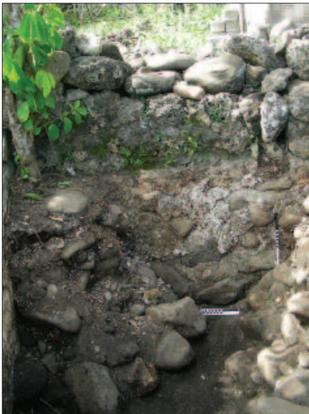
Below: Figure 4: Exposed foundation footing from the Robertson house, Dillon's Bay, Erromango.
